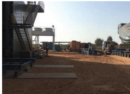
MAN Energy Solutions is supplying two MAN 9L51/60 engines for a newly built power plant in Brikama, Gambia.
