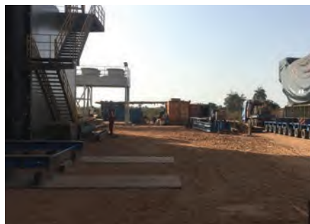
MAN Energy Solutions is supplying two MAN 9L51/60 engines for a newly built power plant in Brikama, Gambia.
