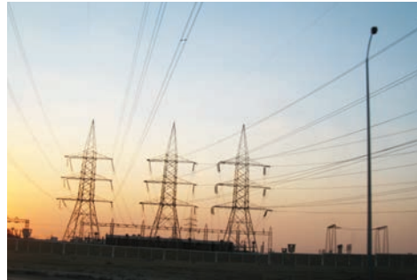
The funding will support a sound electricity infrastructure base.
