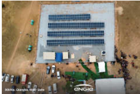
CBEA finances and owns solar mini grids for electrification across the continent.
