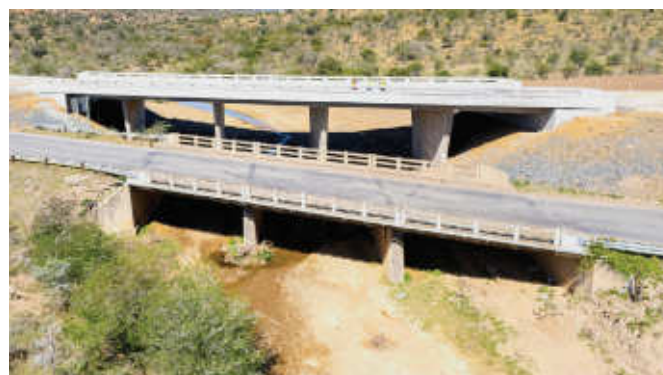
A completely new 65 m long five-span bridge is being built over Mxelo River, with the old bridge to be demolished.
