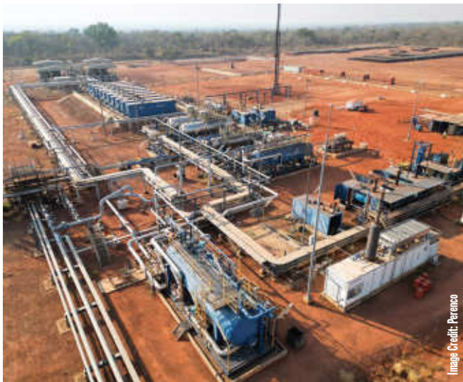
The Moundou Power Station.
