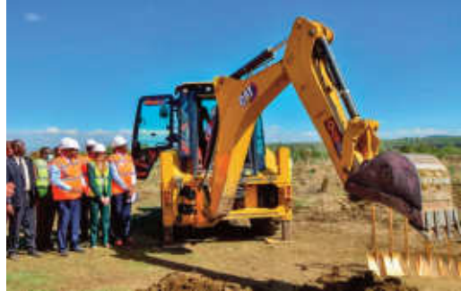
Paul Ngugi, managing director and CEO of GDC, cheers as Deputy President Gachagua breaks ground at the Globeleq site for the construction of a 35MW powerplant.
