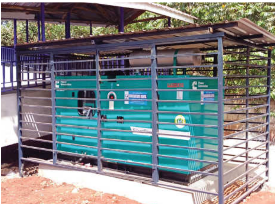
Generators Kenya Limited explained that Cummins and Perkins generators have been standing out due to their reliability, advanced technology and fuel efficiency.
