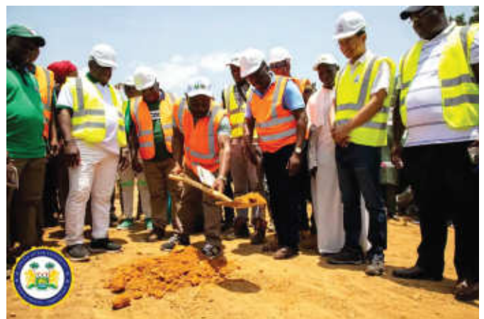
Sod turning for the construction of the Gendema bridge in Sierra Leone.
