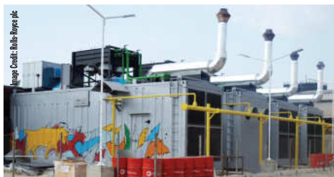
Rolls-Royce mtu 16V4000L32 natural gas gensets installed at IPP producing electricity in 2016 for a food factory in Nigeria.
