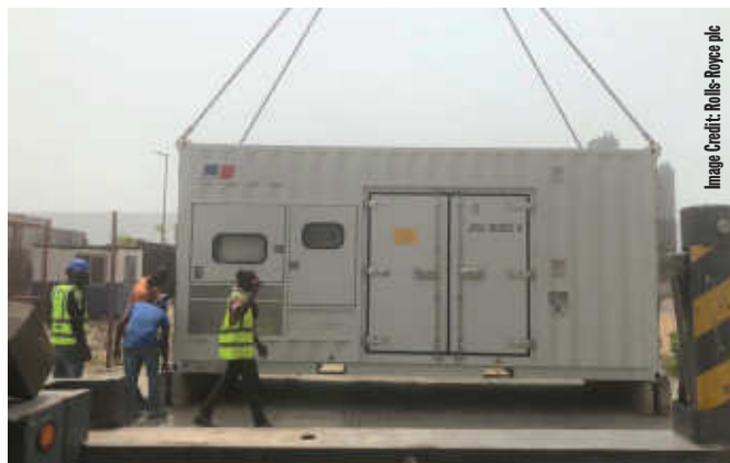
One of the two 1,000kVA diesel generators that power the residential skyscrapers at Azuri Towers in Nigeria.
