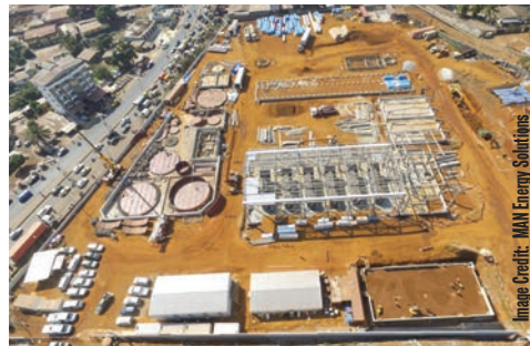
MAN Energy Solutions installs six MAN 18V32/40 engines with a total capacity of 53MW in a power plant in Conakry, Guinea.
