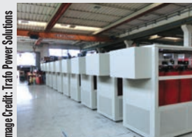
Trafo transformers will be used for a wastewater treatment plant near Vereeniging.
