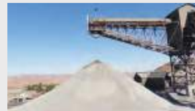
The R-SDR system surrounds the discharge flow on all sides
