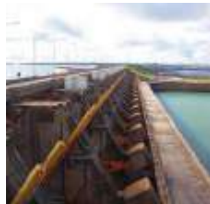
Rusumo falls hydropower plant is expected to attract more sustainable investment
