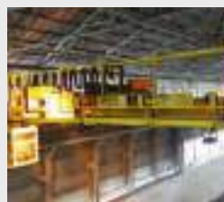
Demag's eight ton electric overhead travel crane
